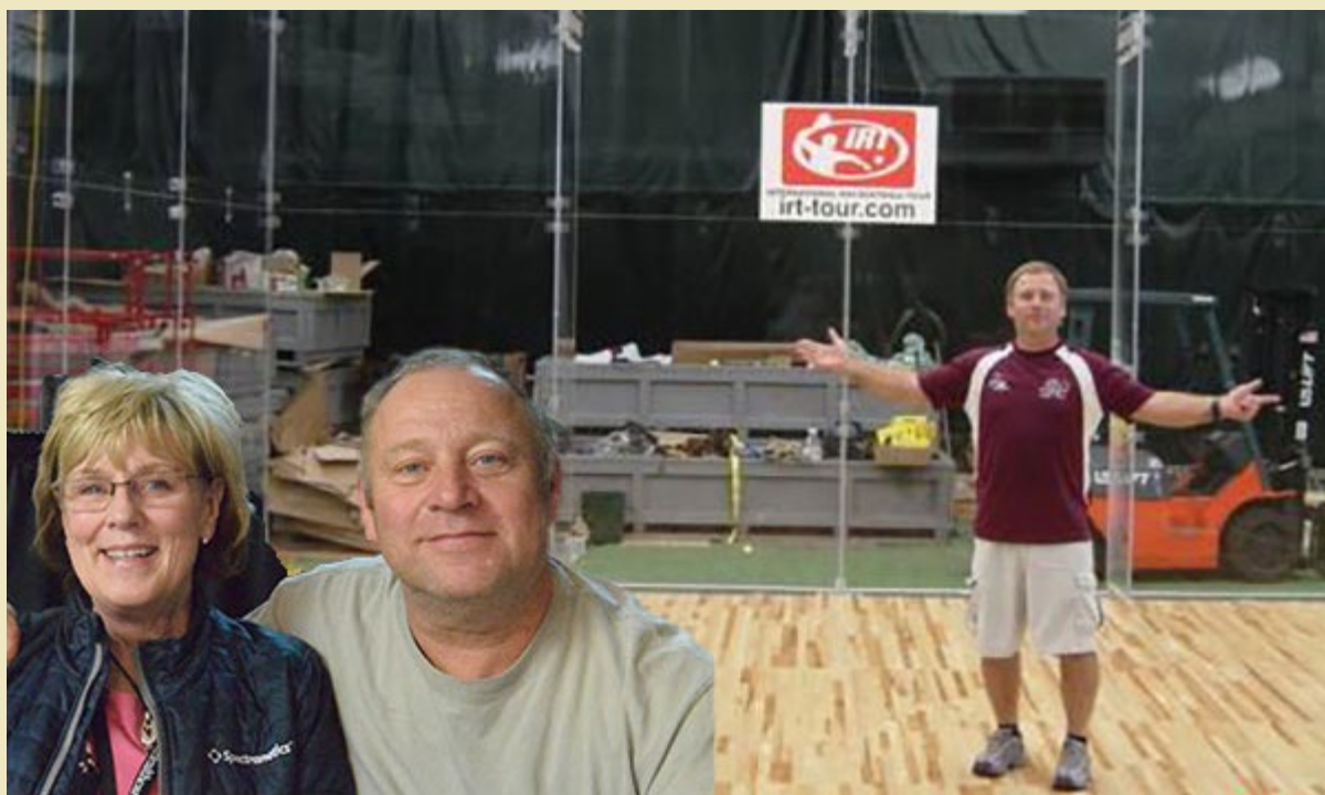
Eddie Meredith has played a pivotal role at the US OPEN for over a decade - by supervising the construction of the portable stadium court each year. His first practice-run was a set-up and tear-down at Lynmar in Colorado Springs in 2007, and he's pictured then and now (inset with wife Mary in Minneapolis last year). 2018 photo by Roby Partovich.
